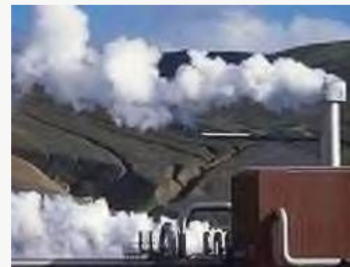
Geothermal energy plant
